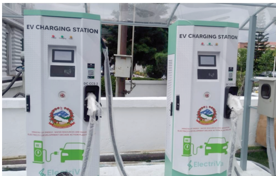
Figure 6: EV charging station installed in the premises of Singha Durbar, Kathmandu. Photo: Rastriya Samachar Samiti
