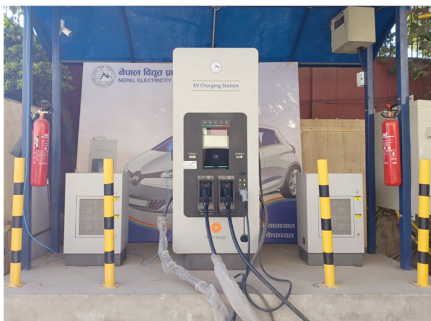
Figure 5: An EV charging station on the NEA premises in Ratna Park. Photo: Diwash Ghimire
